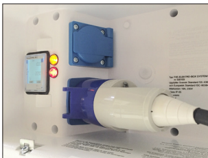
Electricity meter in the mains box with lighting
