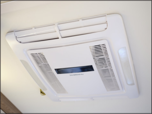
Klimaanlegg – Dometic Fresh Jet FJ2600 (standard Imperial)
