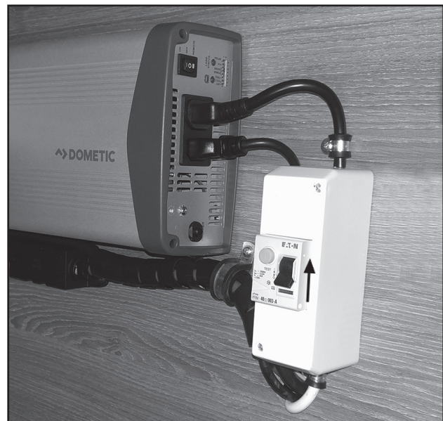
A residual current device is mounted next to the inverter.
