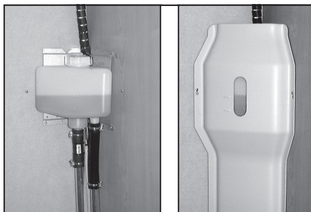
The expansion tank and cover plate with inspection hole.
